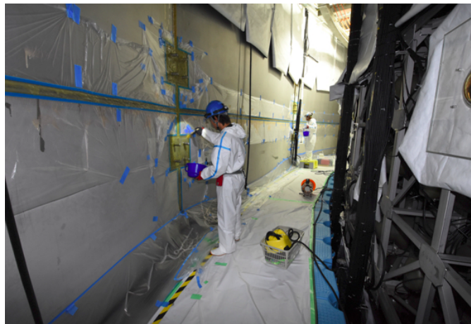
Tank refurbishment in 2018 to stop water leakage
