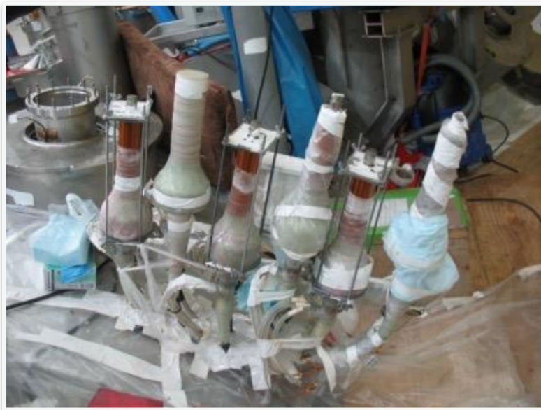
Installation of 24 bus bars on the module and final shaping of the bus bar ends
