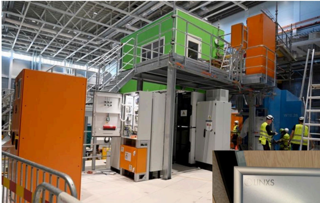
Control room with stairs!
