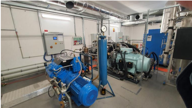
70 m 3 /h and 200 m 3 /h recovery compressors
