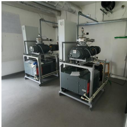
30 mbar helium vapour pumping stations
