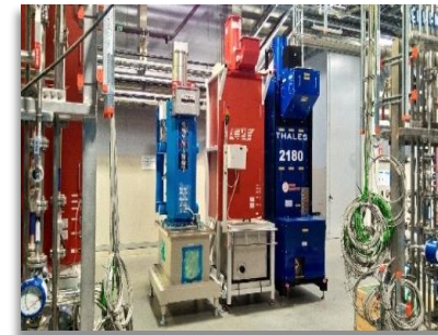
Klystrons at ESS
